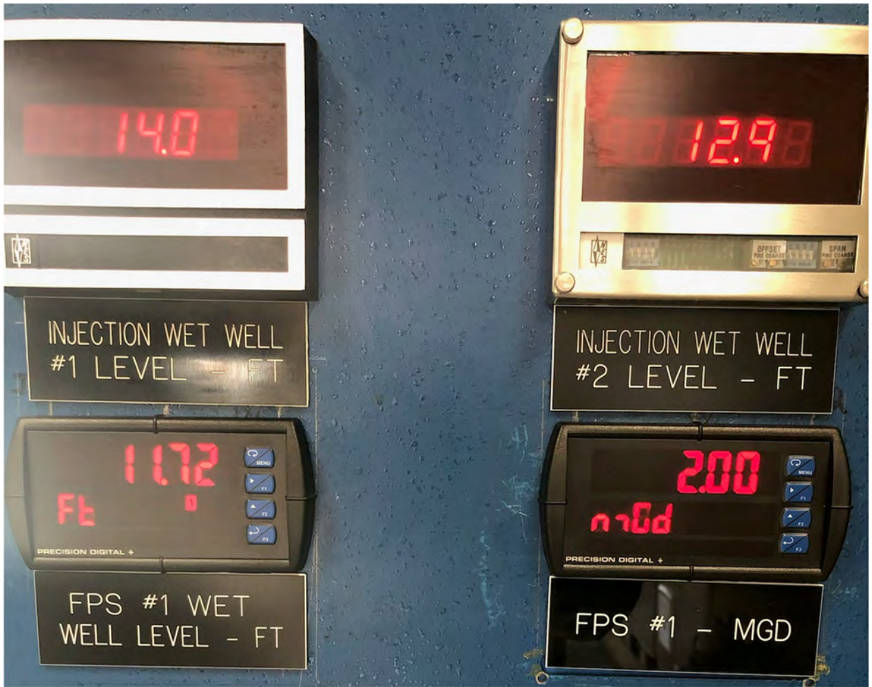
New Local Flow and Level Indicator Display in ER-3 – Filter Pump Station No. 1
