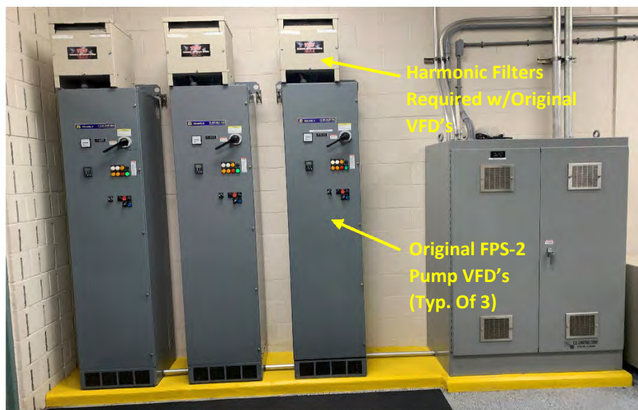
Filter Pump Station No. 2 – Original VFD's
