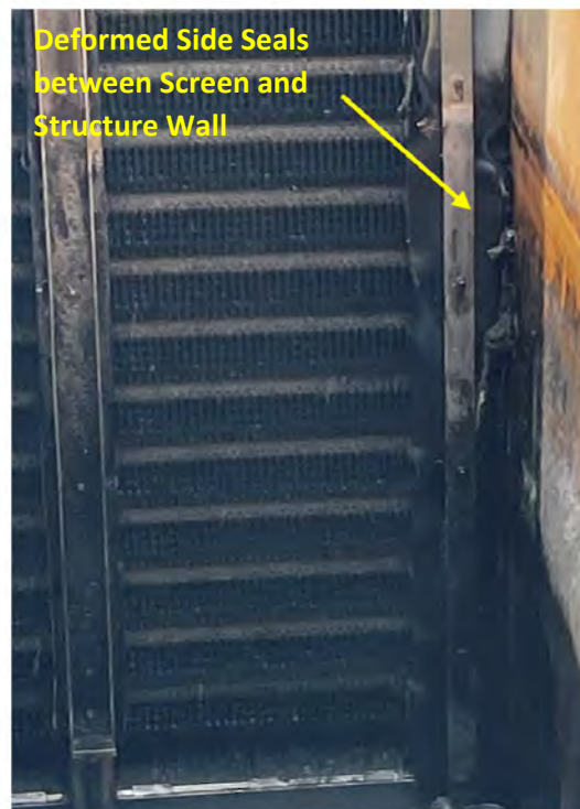
Mechanical Bar Screen – Close-up
