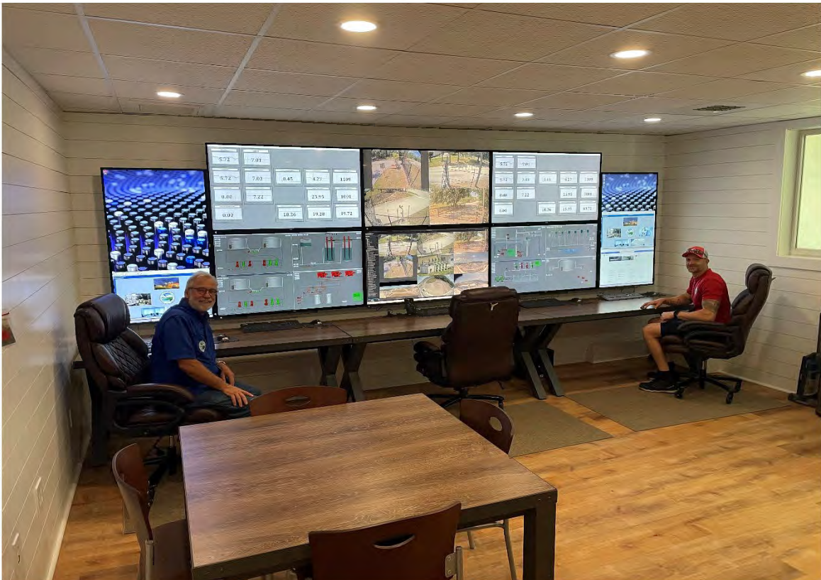
Upgraded WWTP Operations Control Room (with 2 Happy WWTP Operators)
