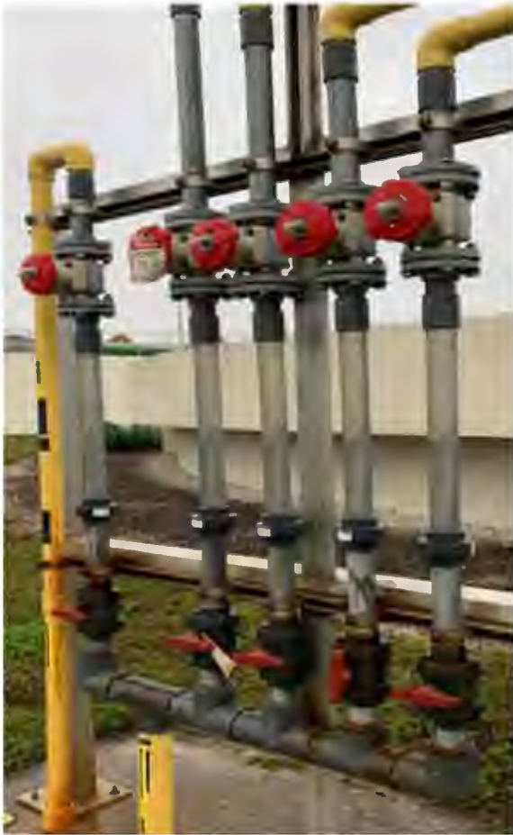
Existing Chlorine Feed Manifold
