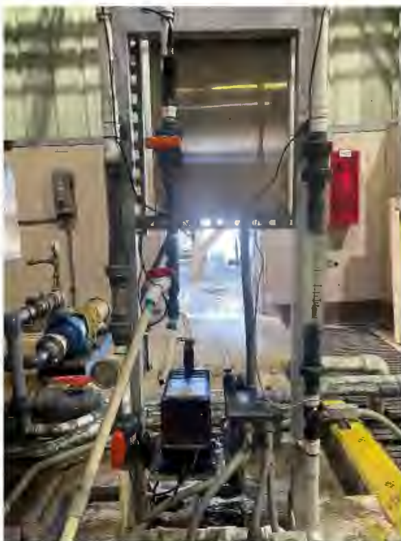
Existing Polymer Make-Up System
