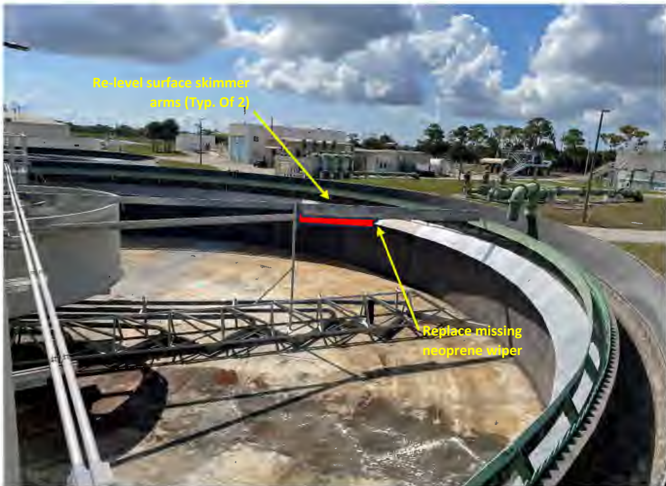
Clarifier No. 3 – Summary of Required Repairs
