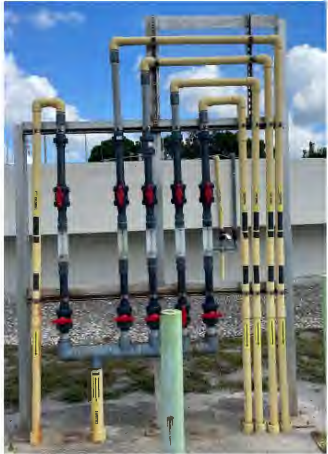
Refurbished Chlorine Feed Manifold
