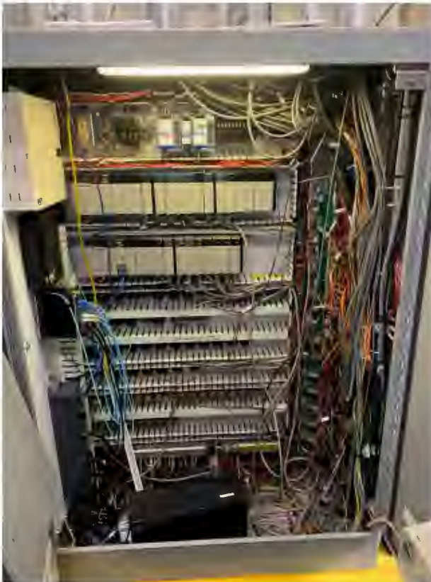
ER-3 PLC Panel 1600 Pre-Work
