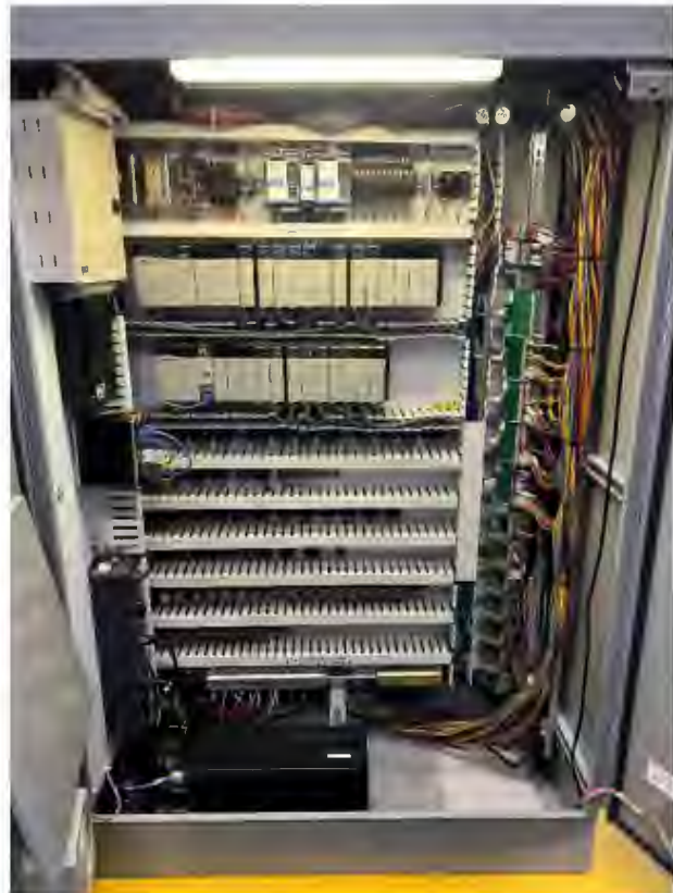
Refurbished ER-3 PLC Panel 1600
