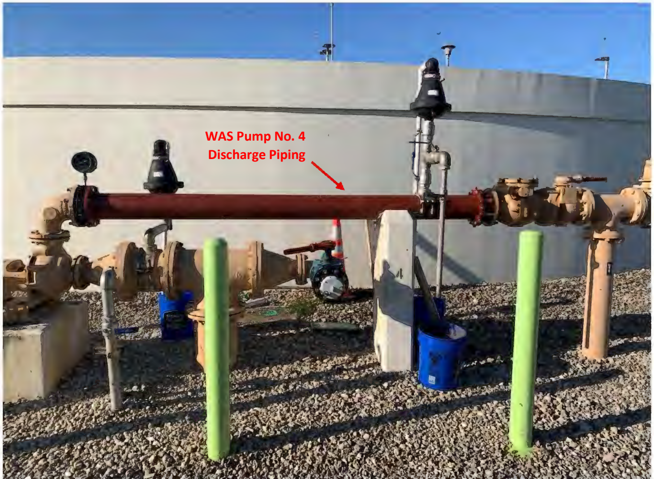
Waste Activated Sludge (WAS) Pump No. 4 and Piping
