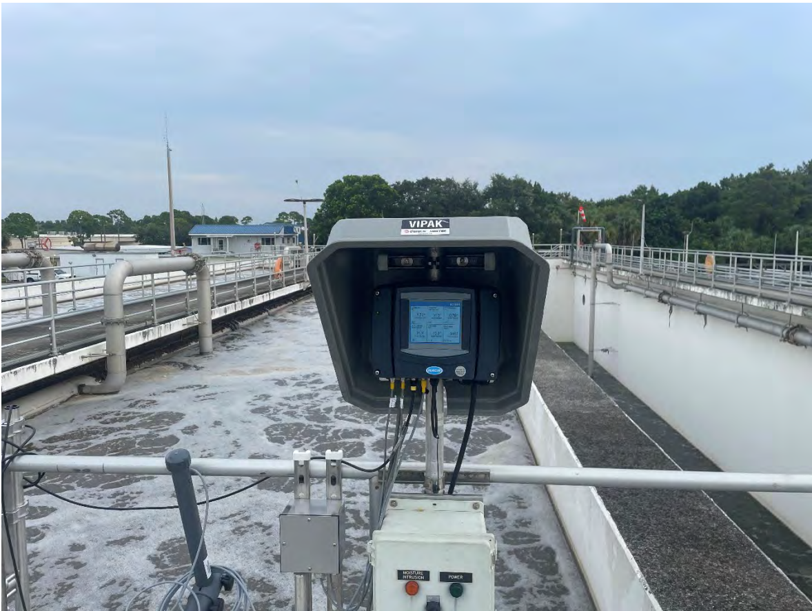
Aeration Basin No. 2 – Process Control Instrument Transmitter
