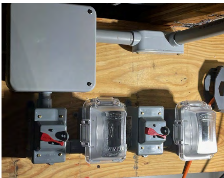
Upgraded Pump Receptacle and Switches
