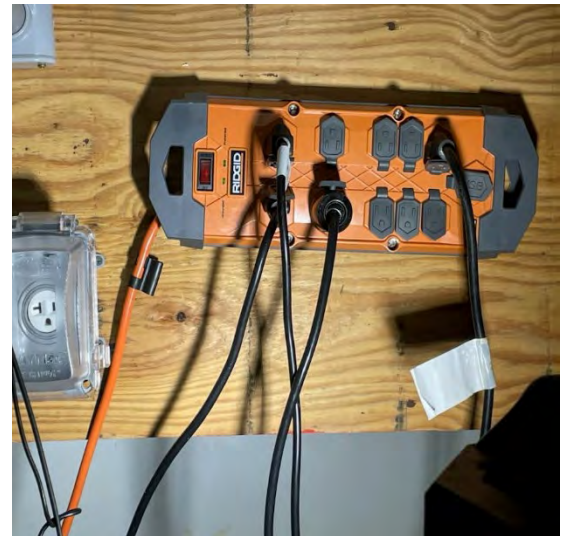
Existing Receptacle Box
