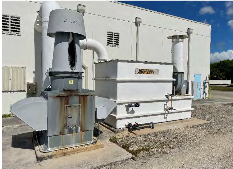
Chlorine Building Air Scrubber Unit
