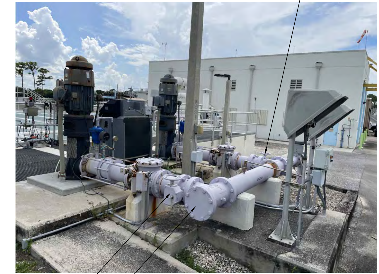
VALVE 13012 TIE TEMPORARY NPW PIPING FROM STABILIZATION POND A INTO EXISTING 8" NPW PIPING
