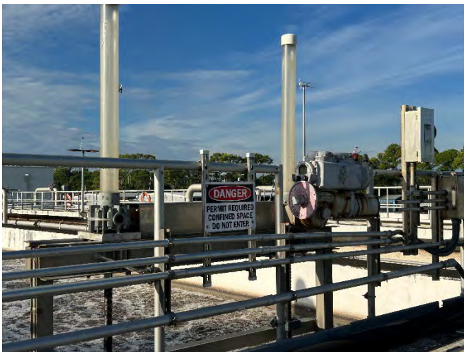
Existing Motor Operated Gate Actuator
