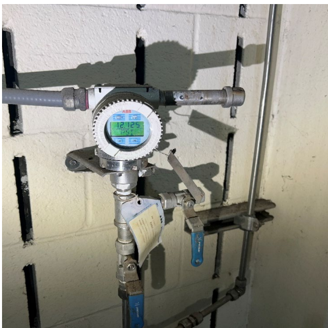
Original Process Air Pressure Transmitter
