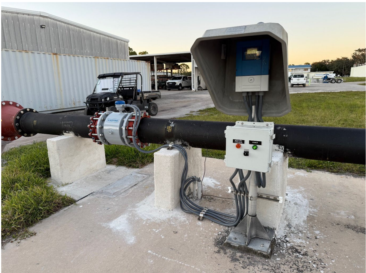
IQ-512 Lift Station – Replacement Inline Magnetic Flow Meter and Transmitter
