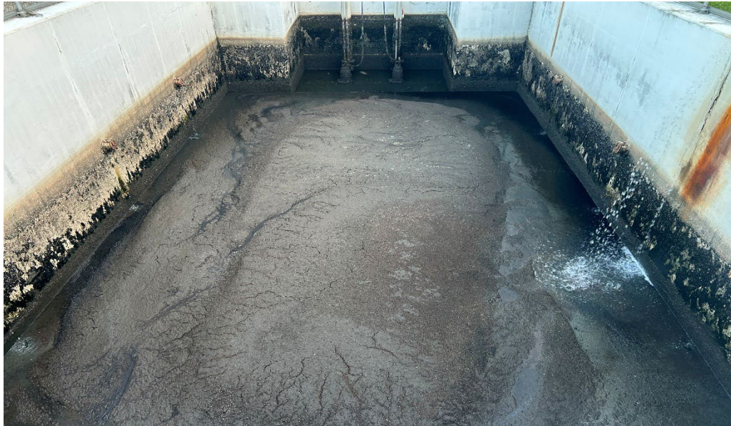
Filter Backwash Basin – Pre Cleaning
