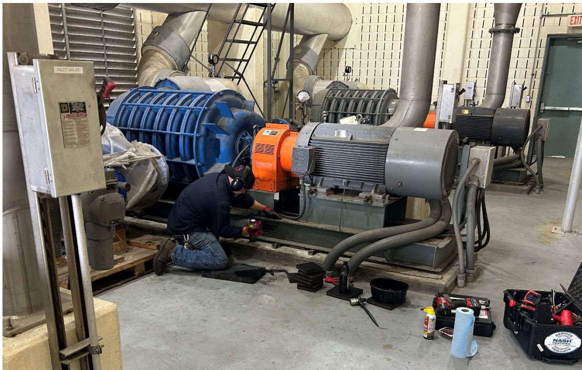
Main Process Air Blowers – Annual Maintenance and Repairs
