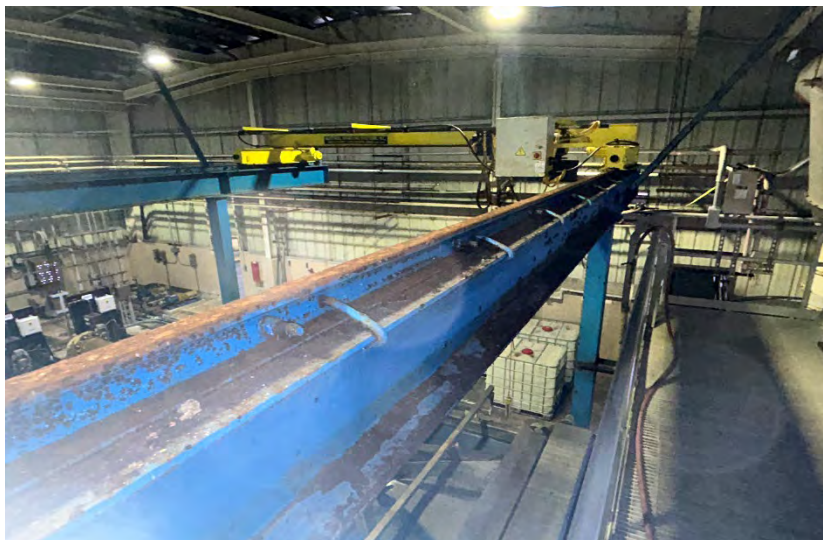
Solids Dewatering Facility OH Crane – Pre-Work
