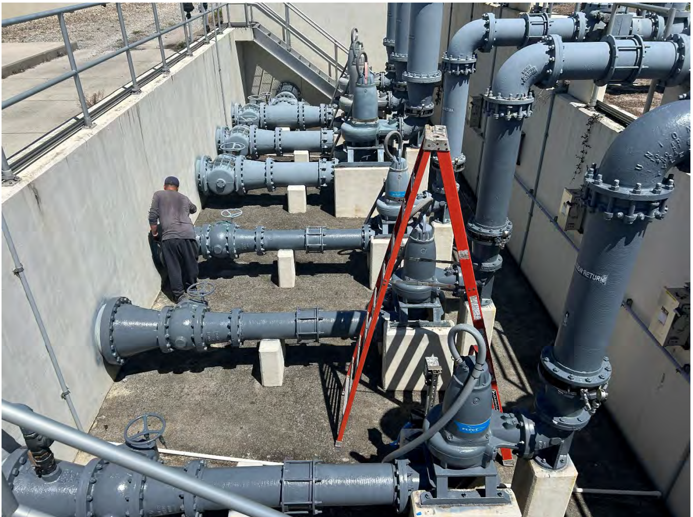
Equalization Return and Mixing Pump Station
