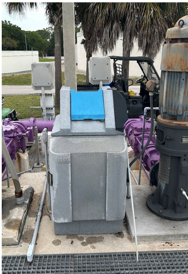
Existing Composite Sampler Unit
