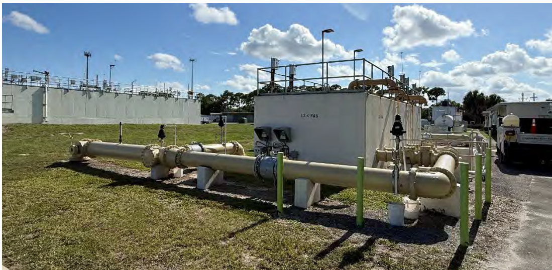
Return Activated Sludge Pump Station
