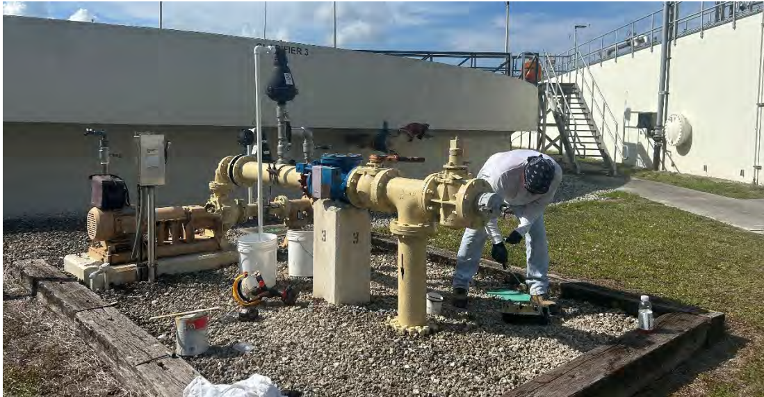
WAS Pump Station No. 3
