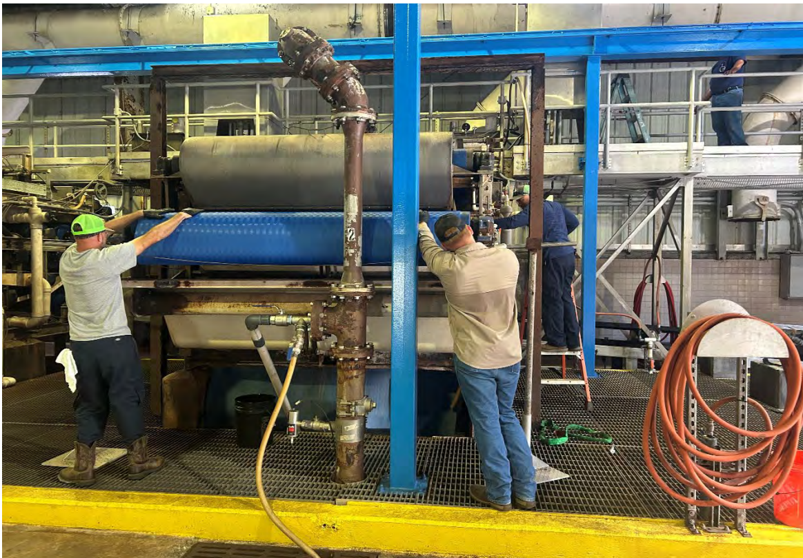
Belt Filter Press Unit – Belt Replacement Maintenance
