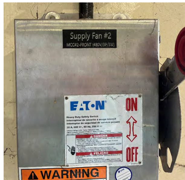
Electrical Panel Labelling Example
